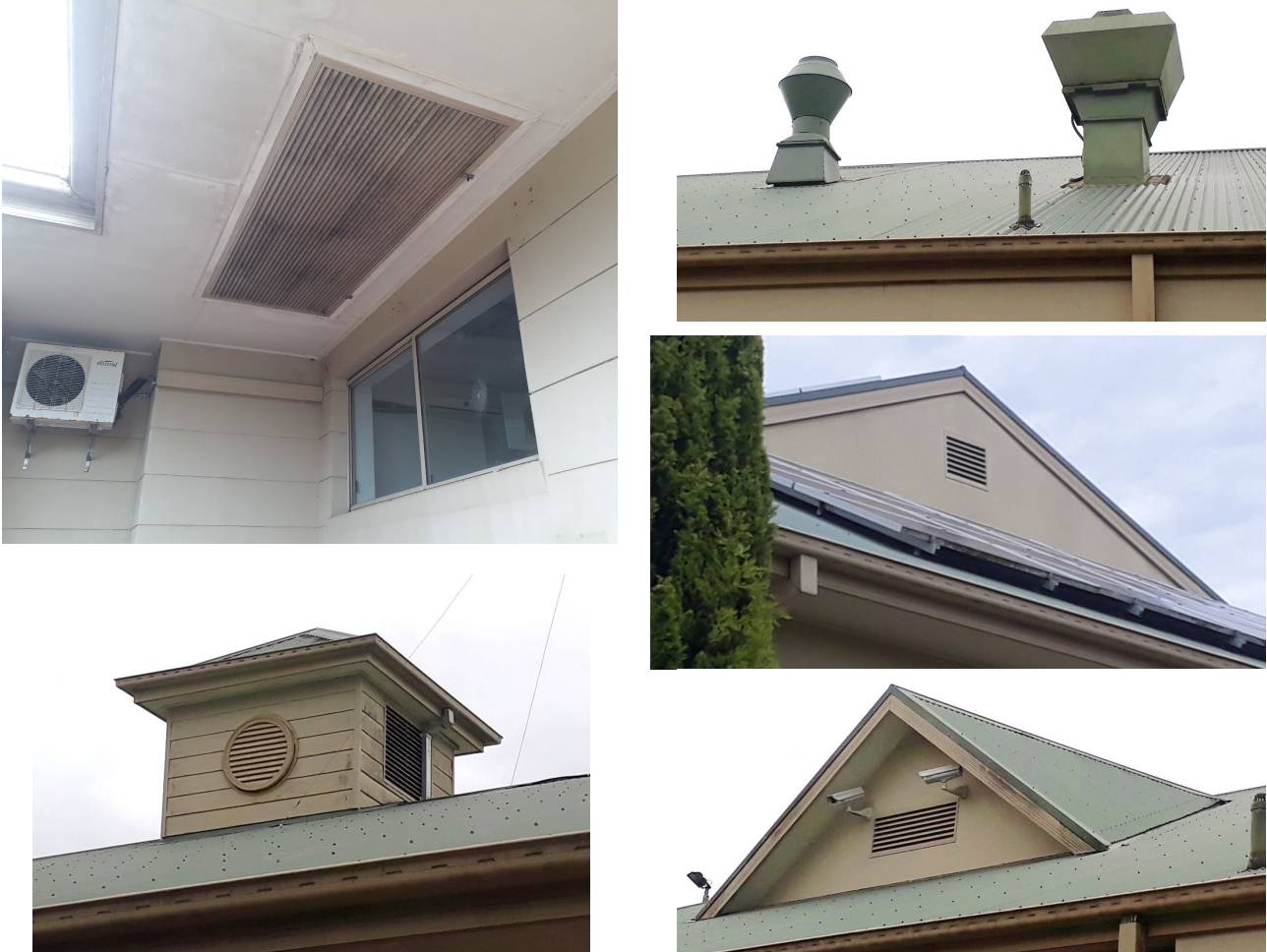
Figure 2: Examples of vent openings that appear to have no ember protection.
