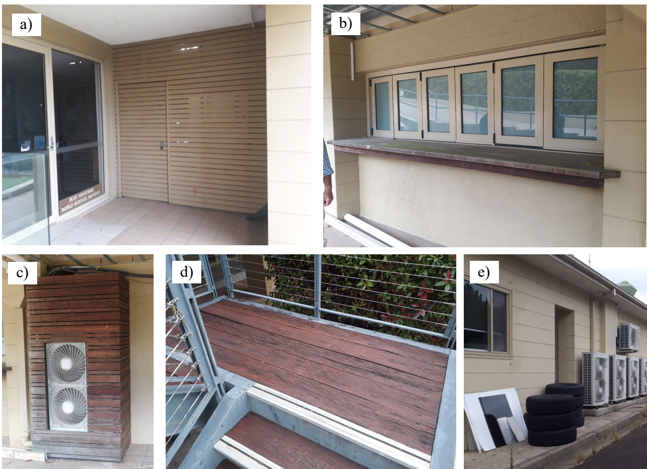
Figure 5: Combustible materials posing a hazard to the building. Labels a–e correspond to items in the list near the top of this page.
